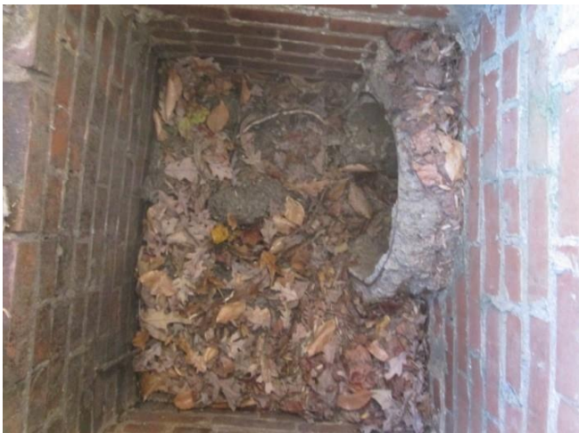
Catch Basin with heavy debris before cleaning
