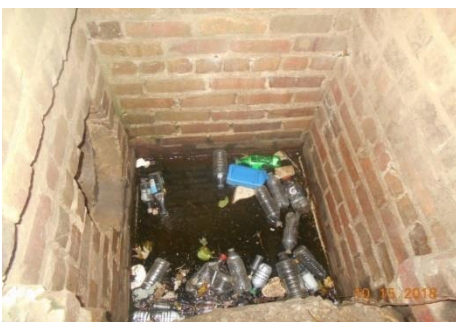
Catch Basin full of debris before cleaning
