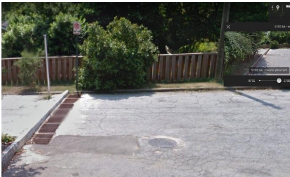
Street view and CCTV show 7 grated inlets connected to a sanitary sewer
