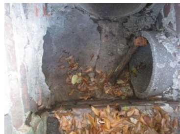
Catch Basin before cleaning
