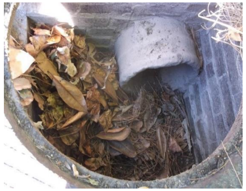
Catch Basins with heavy debris
