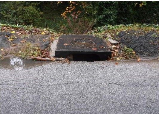
Catch Basin filled with debris
