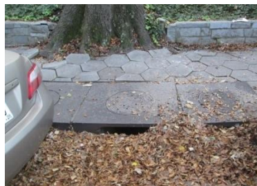
Debris at street level
