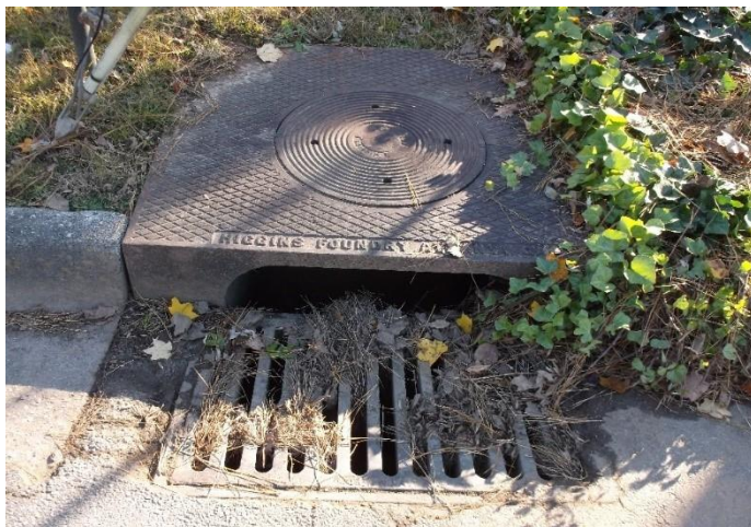
Catch Basin before cleaning
