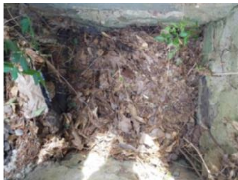
Once cleaned discovered root infiltration
