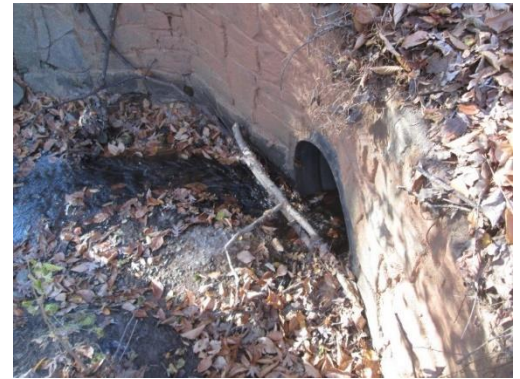
Failing headwall with debris before cleaned
