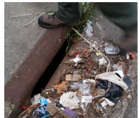
Catch Basin and grates before cleaning
