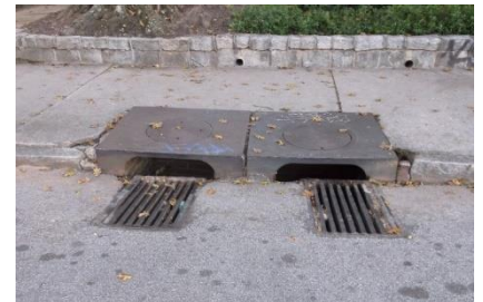
Strong smell of sewerage.
