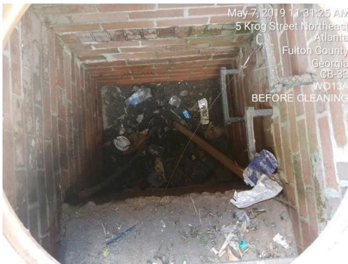
Catch Basin before cleaning
