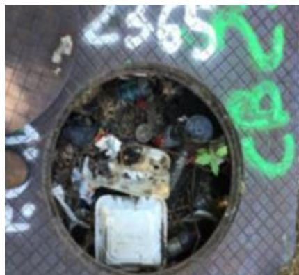
Catch Basin before cleaning
