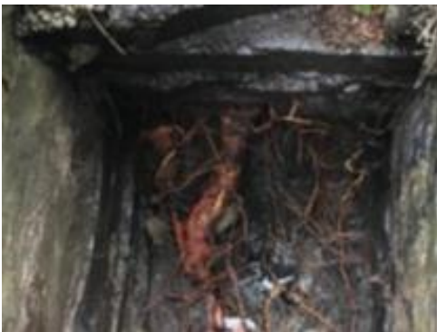
Heavy leaf and debris accumulation in Catch Basin
