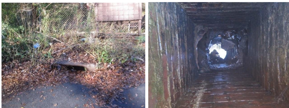
Catch Basin with heavy debris and holding water
