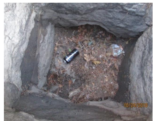
Catch Basin before cleaning
