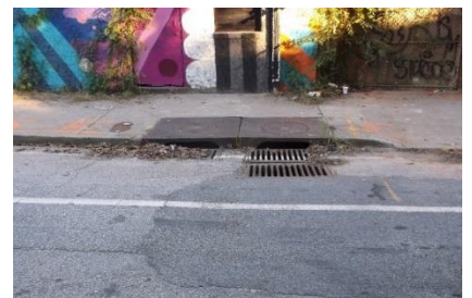
Catch Basins with grates holding water and debris; strong smell of sewerage.
