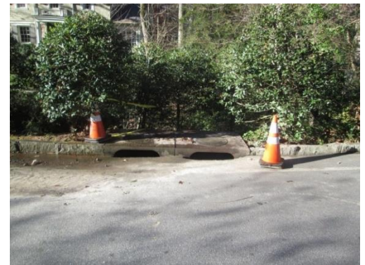
Catch Basins with compromised throats
