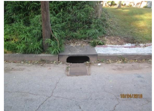
Catch Basin with grate at street grade
