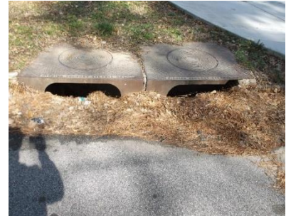
Catch Basins at street level severely compromised with leaf debris
