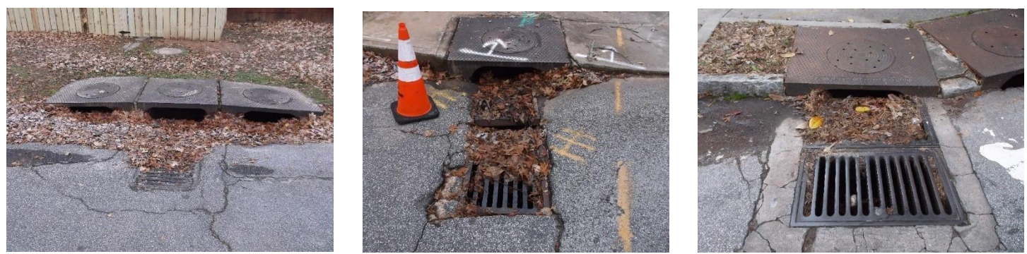
Catch Basin and grates with debris at street level before cleaning
