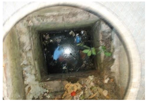
Debris and holding water
