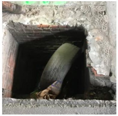
Catch Basin comprised and dysfunctional due to debris
