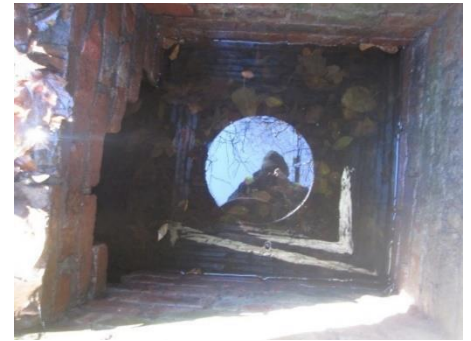
Inlet with heavy debris and holding water
