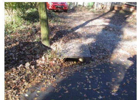
Inlet with heavy debris and holding water
