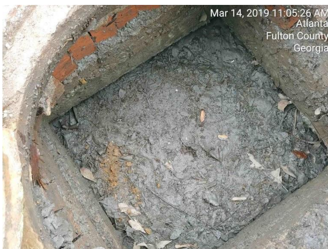
Catch Basin before cleaning
