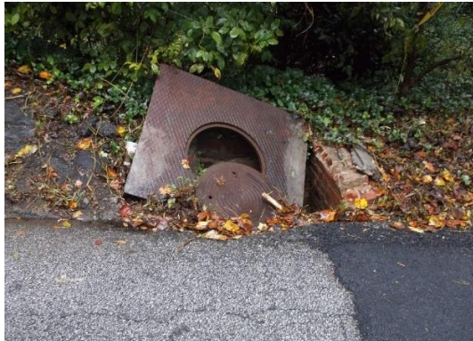
Damaged Catch Basin top
