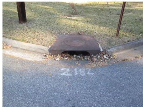
Catch basin with debris at
