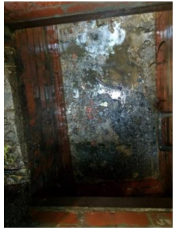
Catch Basin before cleaning
