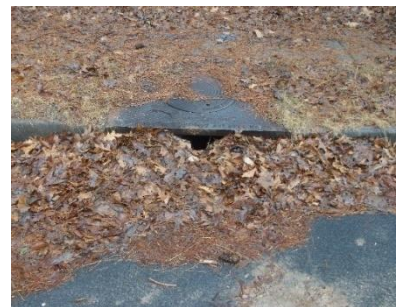
Clogged catch basins
