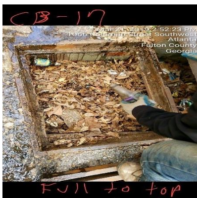
Catch Basin full to the top with leaf debris and trash
