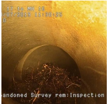
CCTV abandoned due to roots in pipe
