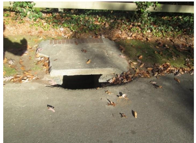
Catch Basin top – no access/lid
