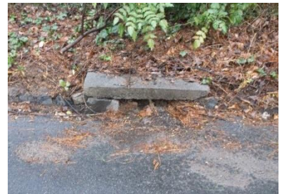
Damaged catch basins
