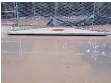
Catch Basin with street ponding
