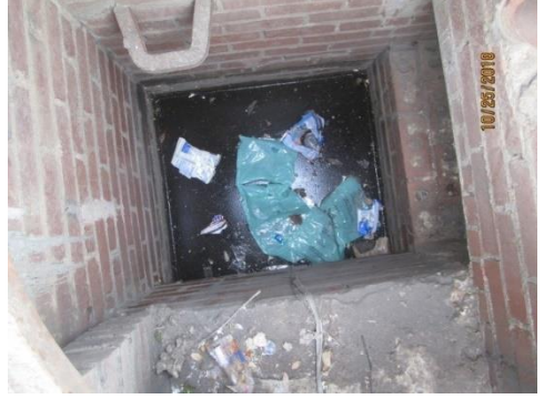
Catch Basins with heavy debris
